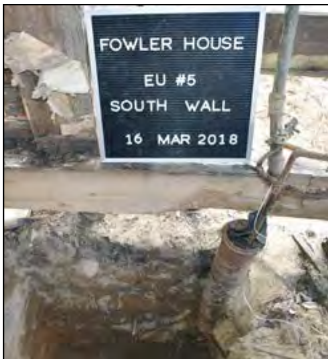
Electrical submersible pump identified along the south wall of the Fowler House.
